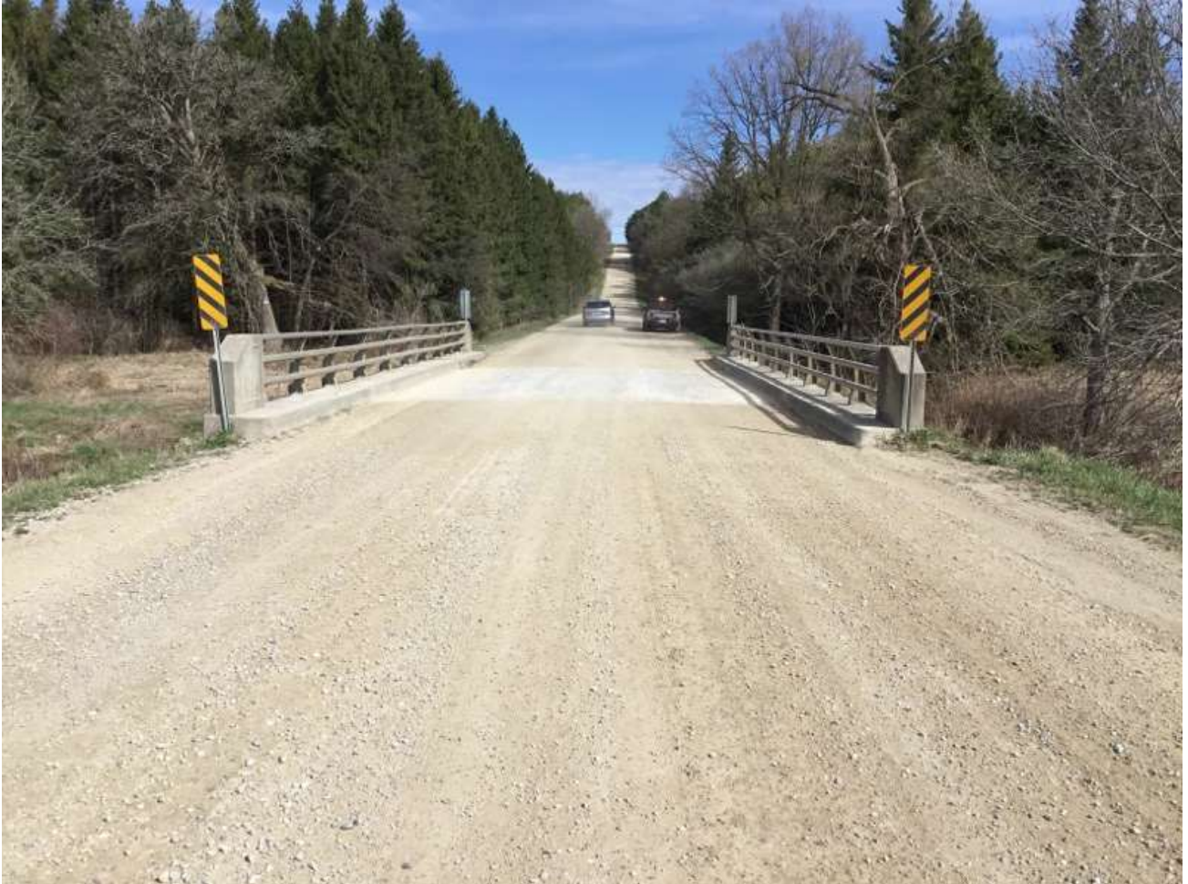
Figure 4: Bridge on 10th Line In Fair Condition (40) as of last assessment date
