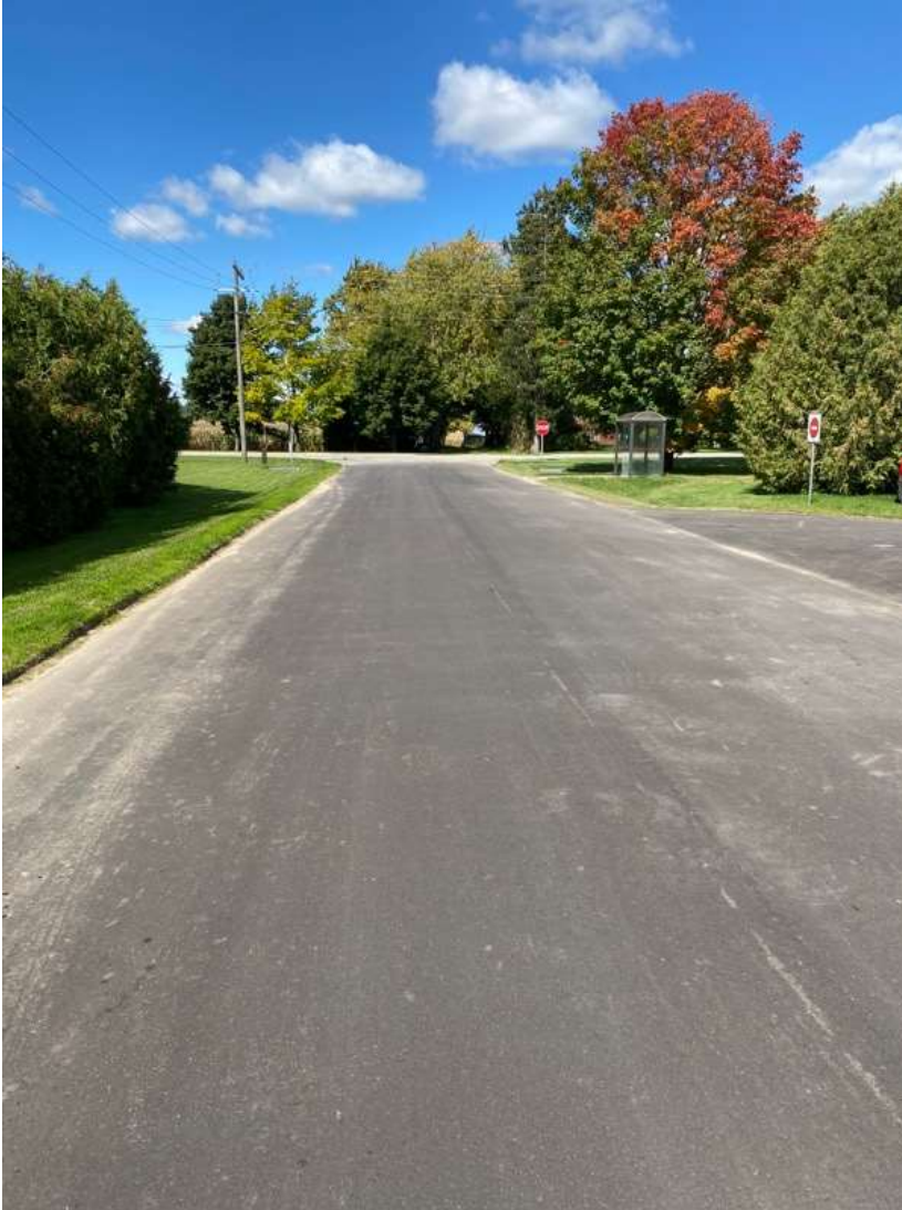
Figure 1: An example of a road (0405-01) in very good condition as of the last assessment date.
