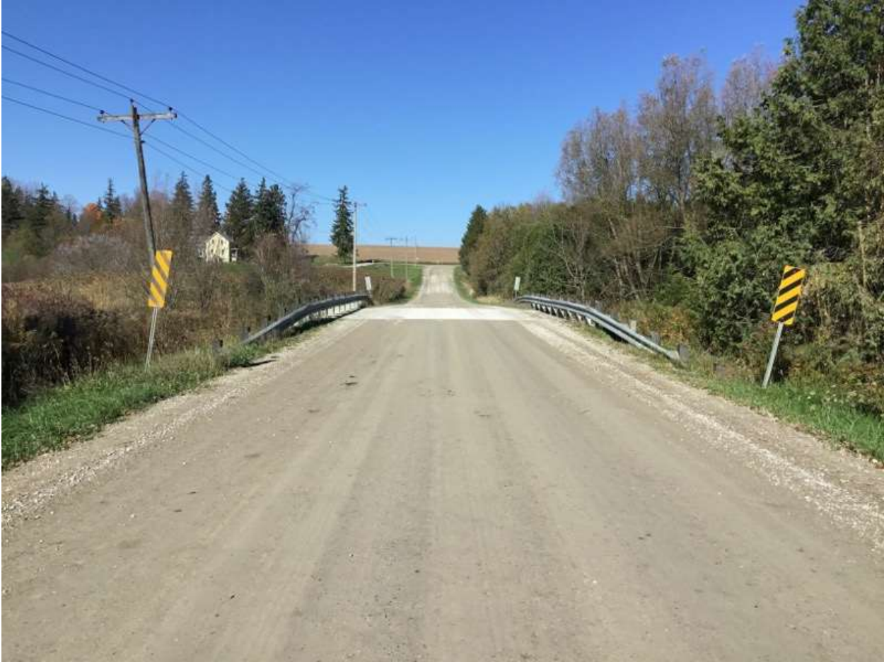
Figure 6: Bridge on 10th Line in Very Good condition as of last Assessment Date
