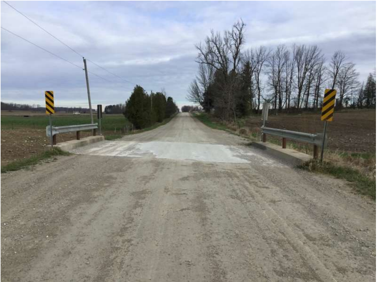
Figure 5: Bridge on 14th line in Good Condition (60) as of last Assessment date
