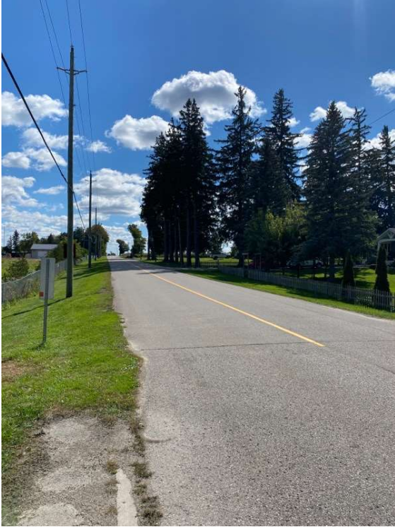
Figure 2: An example of a road (0479-00) in good condition as of the last assessment date.
